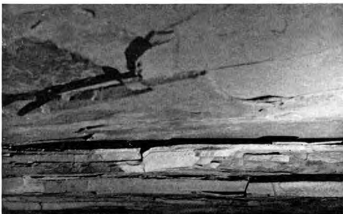
1½ inch sag in cantilevers, Poorfarm Cave, W. Va. Vertical joints separate the rock beams into cantilevers of various lengths.
